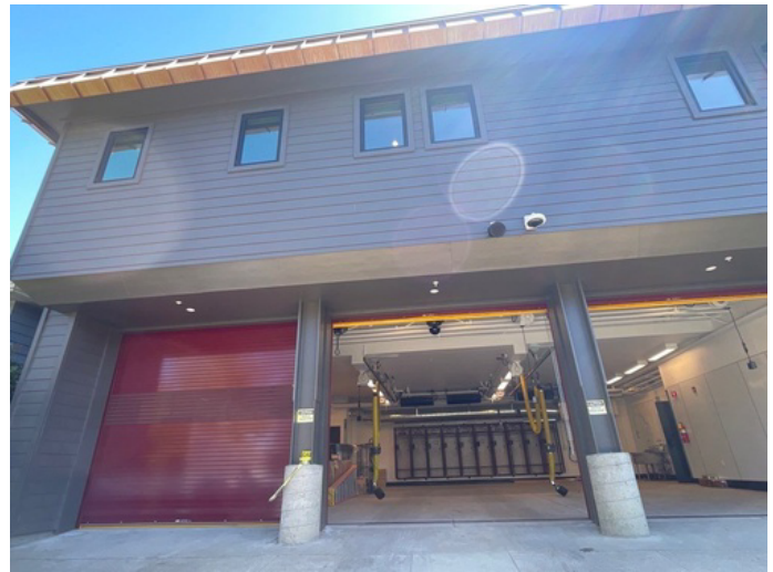
Includes painting eaves, window and door casings, and posts on building. Does not include roll up doors.
